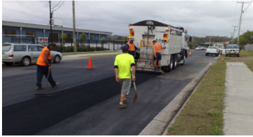
Asphalt overlay in progress, via Ausroad TM HD Series Road Maintenance Unit
