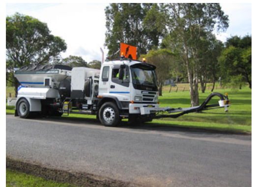
Wyong Shire Council's (NSW) 4m 3 Jetpatcher ® unit, purchased in April 2008. Jetpatching in progress.
